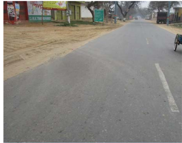
2. Worn out pavement marking: S – 5 (0+200 to 0+400 Centreline)
