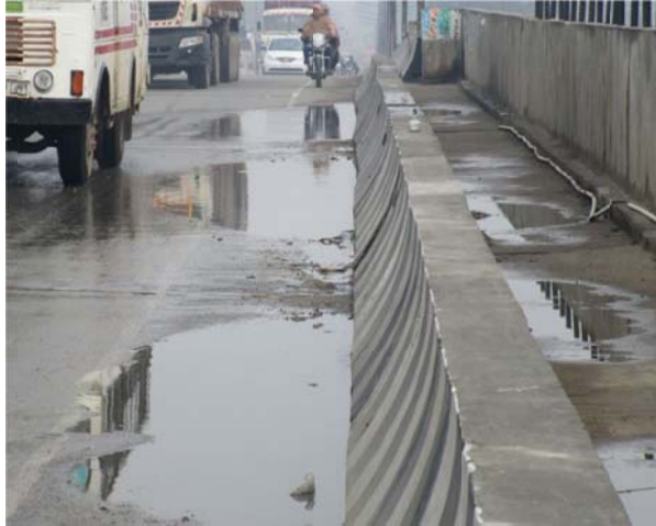
1. Drainage water stagnant on deck slab (R.O.B): S3 - (5+200 R.O.B)
