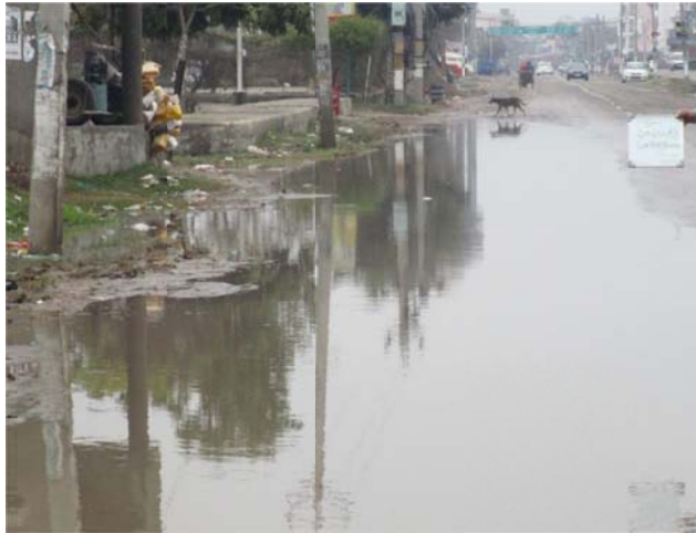
1. Water ponding on pavement : S1 - (0+800 R.H.S)
