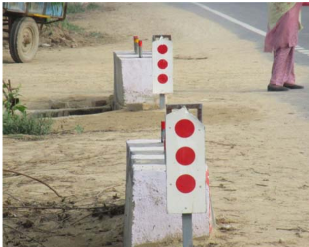
6. Culvert Board Damaged: S4 - (23+170 L.H.S)
