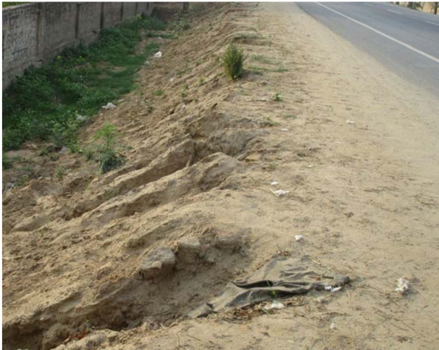
1. Rain Cuts (Improper embankment slopes): S4-(0+150 to 0+200 L.H.S)
