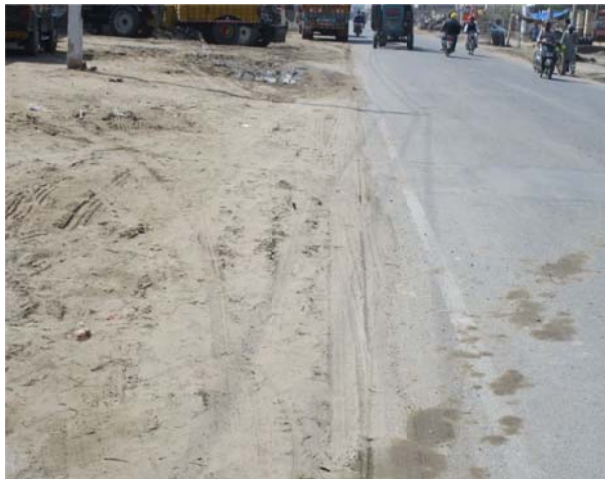
3. Paved & Earthen shoulder not maintain: S3 - (124+800 R.H.S)
