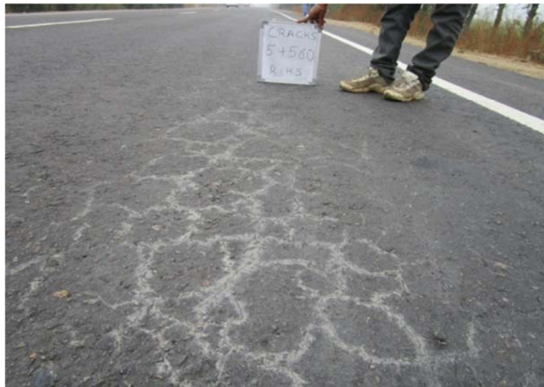
Figure 2-1 : Sector S2 – Cracking – km 5+560 R.H.S
