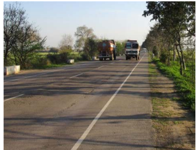
4. Lack of grading in shoulder part S1 - (3+400 R.H.S)
