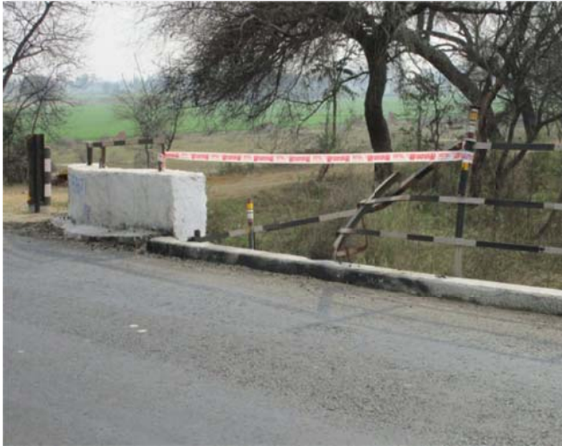
3. Bridge safety railing damaged: B8 - (20+600 R.H.S)
