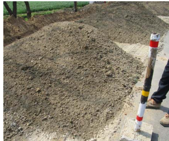
3. Crushed material (work in construction): S4 - (16+690 L.H.S)
