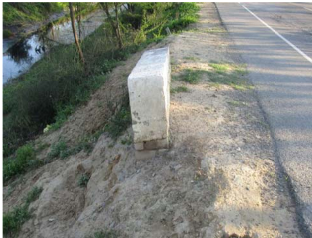
3. Parapet wall is inclined and rigid foundation is required: S1 - (6+200 L.H.S)
