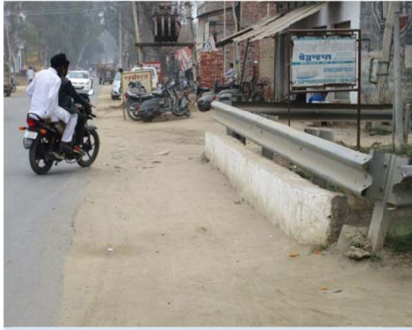
1. Parapet wall Damaged/not painted: S – 5 (25+000 R.H.S)
