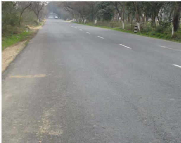
1. No Pavement Marking: B8 - (18+105 L.H.S)
