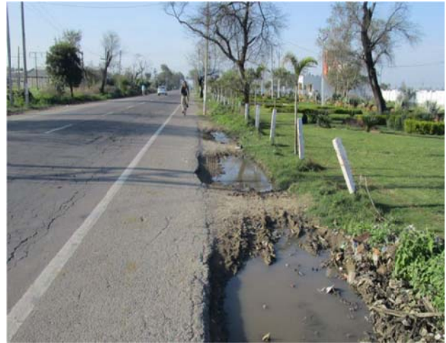
2. Potholes in shoulder Area: S1 - (4+7000 L.H.S)
