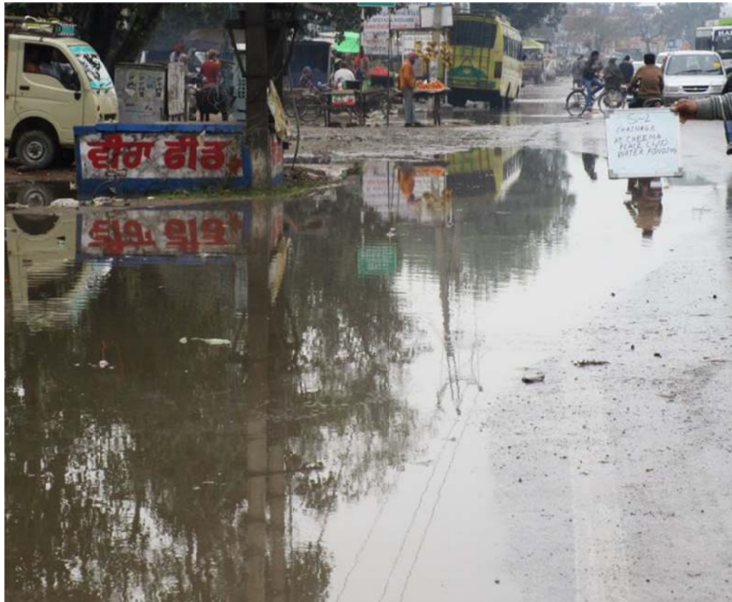
1. Drainage water adjoining pavement edge: S2 – K 54+010 L.H.S)
