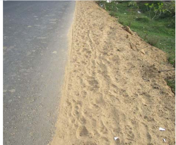
4. Improper Compaction: B8 - (25+750 B.H.S)
