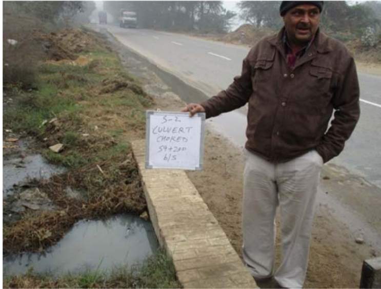
Figure 2-3 : Sector S2- Culvert clogged - Km 59+200 B.H.S
