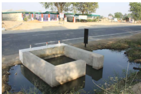
Figure 1-8 : Sector S2- Culvert clogged - K 71+800
