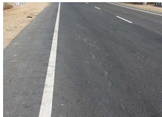
Figure 1-5 : Sector S2 – Cracking – km 7+300
