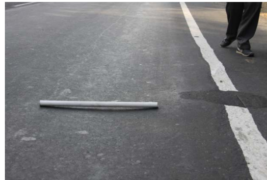
Figure 1-3 : Sector S2 – Rutting – k79
