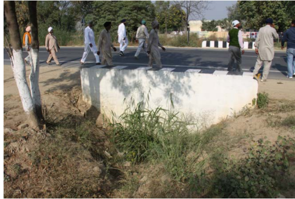
Figure 1-9 : Sector S2- Culvert clogged - K 77+350
