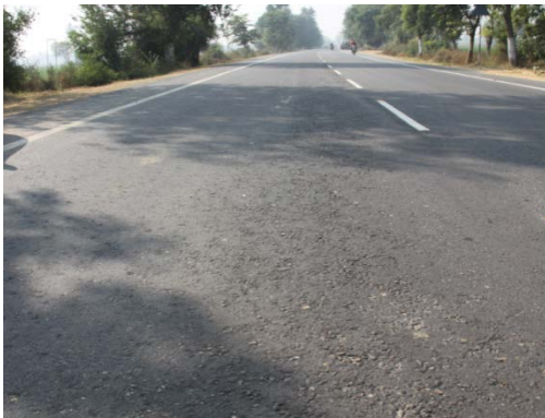
Figure 1-2 : Sector S2 - Raveling km 16+940
